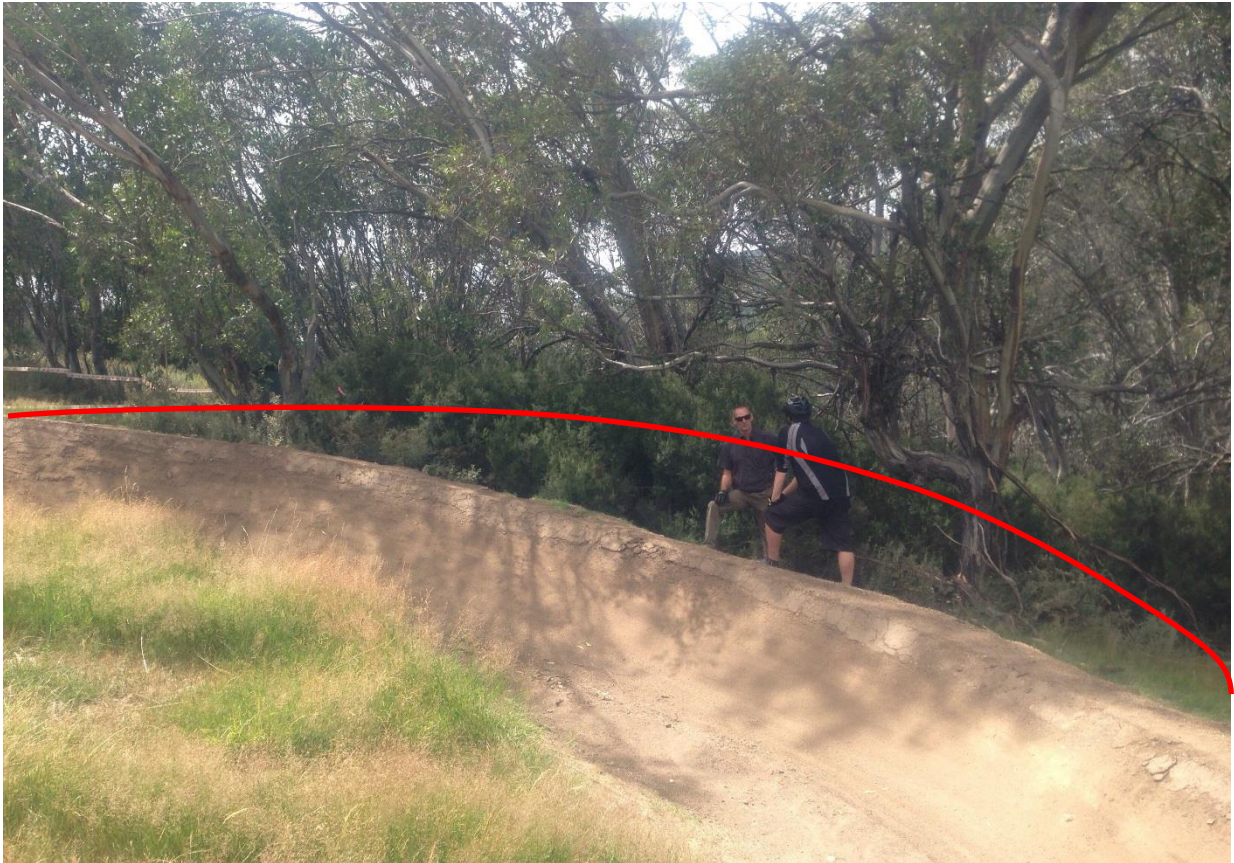
Photo 17: Section 8 involves extending the corner further into the regrowth subalpine woodland tree island so that the corner is off the ski run.
